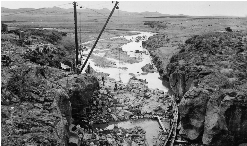
Figure 7. Construction of Sullivan Lake and Dam near Chino Valley (Call Number: dam132pq). Photo courtesy of Sharlot Hall Museum, Library and Archive, Prescott, Arizona
