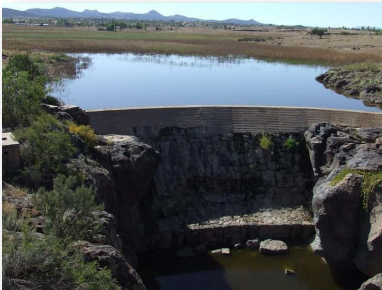
Figure 7.6. Low concrete dam that forms now-ephemeral Sullivan Lake. Dam, about 115 feet wide, is set into the head of a narrow steep-walled canyon cut into basalt. The dam marks river-mile zero on the Verde River, although the uppermost perennial reach now begins about a mile below the dam. View is westward. Photo by E. W. Wolfe,
