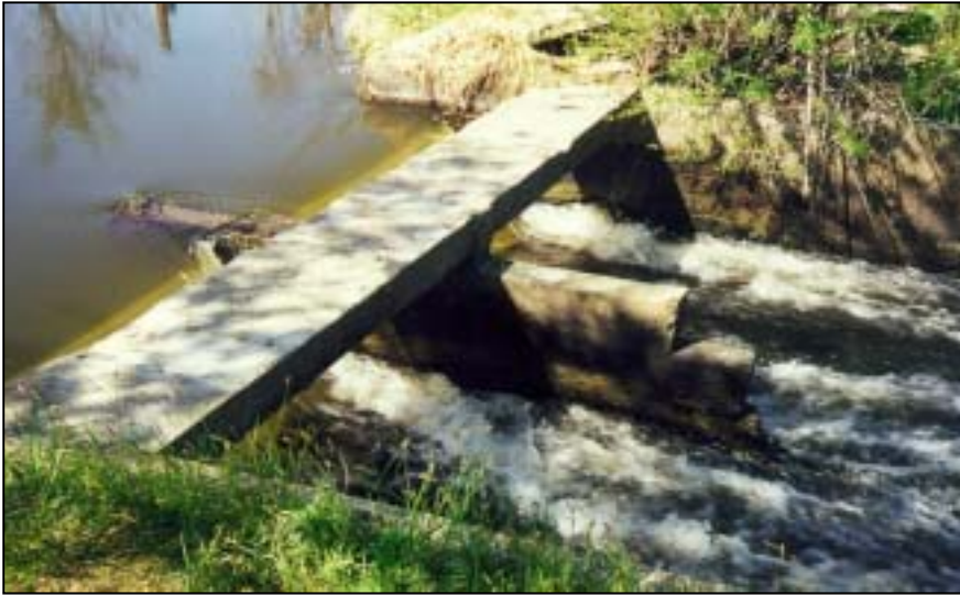
Aging irrigation water control structure
