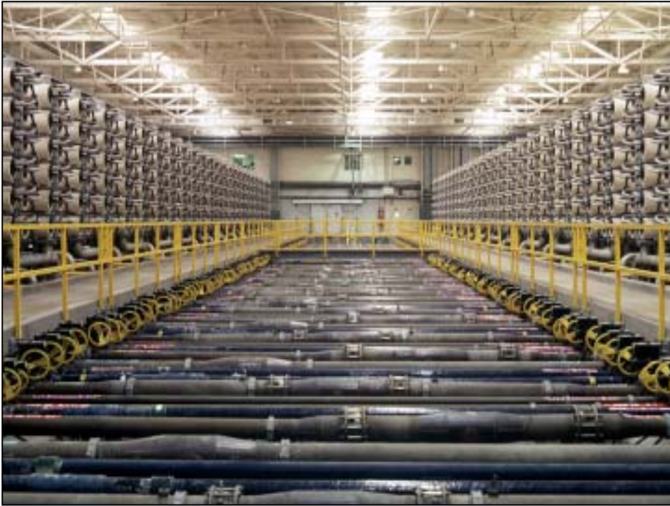
Reverse osmosis water treatment plant
