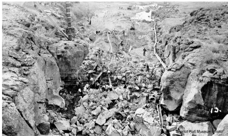
Figure 2.14 —A 1936 photo showing the early construction phase of excavating basalt rock for the base of Sullivan Dam. Perennial flow from Del Rio Springs was routed through a sluice box visible on the right side of the rock cut. (Photo courtesy of the Sharlot Hall Museum, Prescott, Arizona.)
