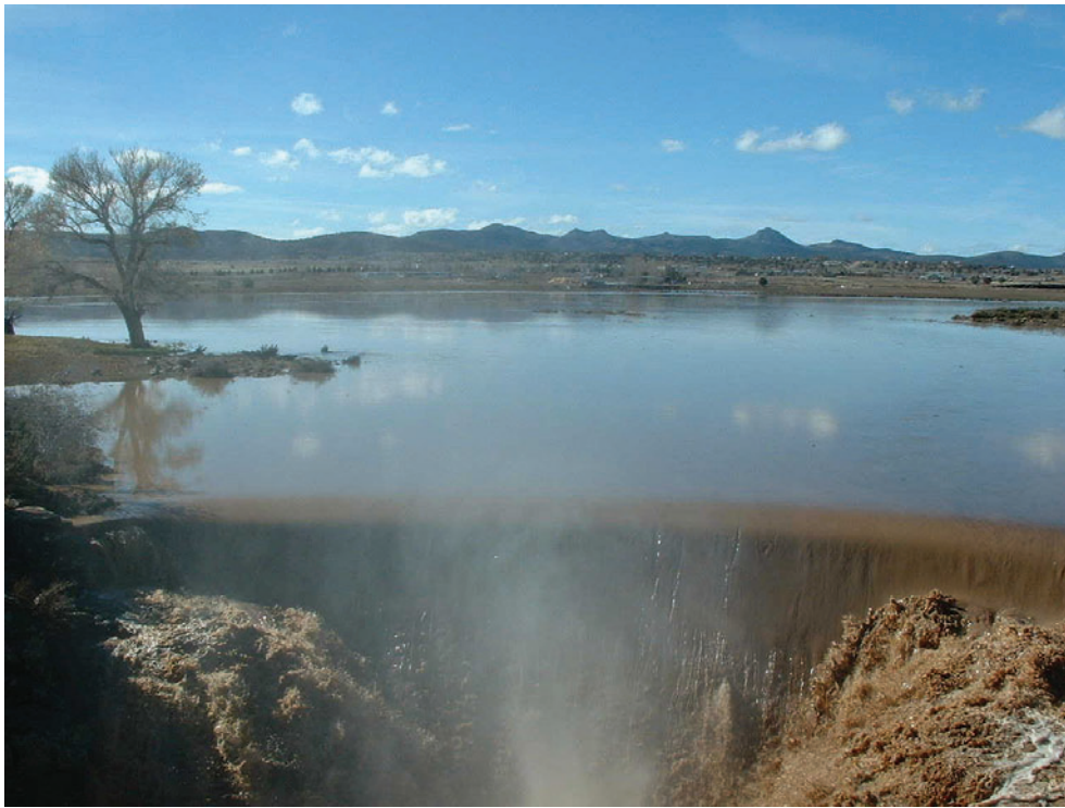
Figure 9.8 —Flow over Sullivan Dam during spring runoff, 2005. (Photo by Alvin L. Medina.)
